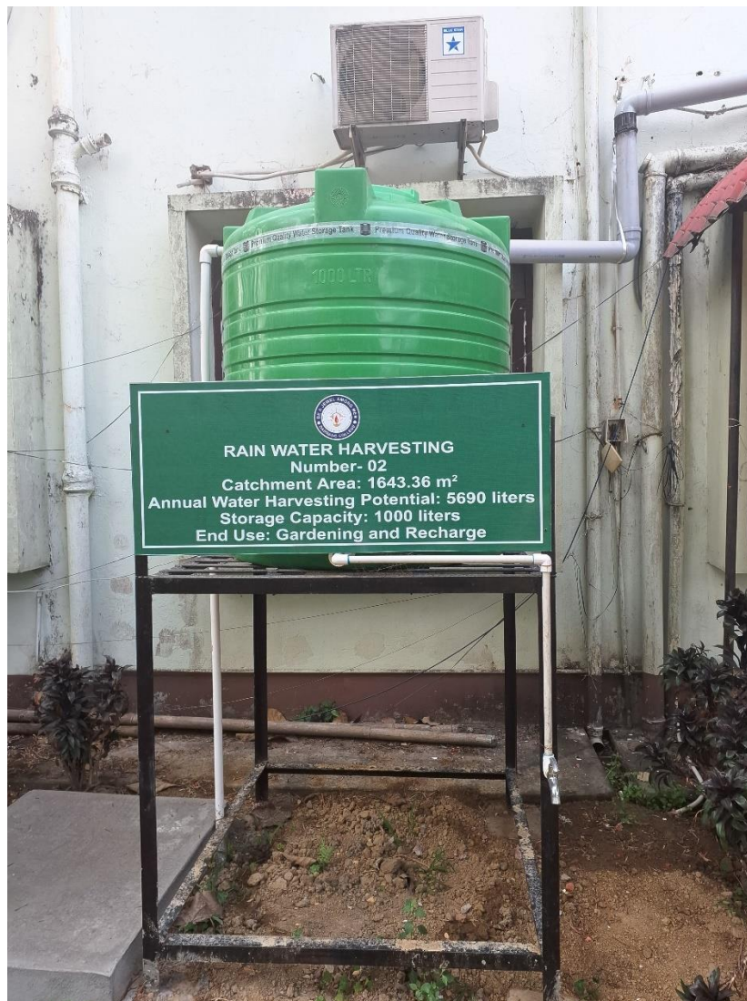
Fig. 14 Rain water harvesting system installed in the College
